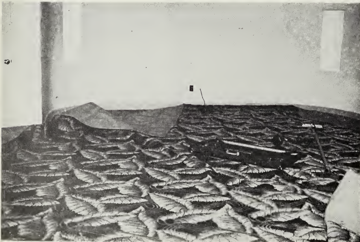
The proper installation of theatre carpet is a precise job, and requires services of a trained expert.
